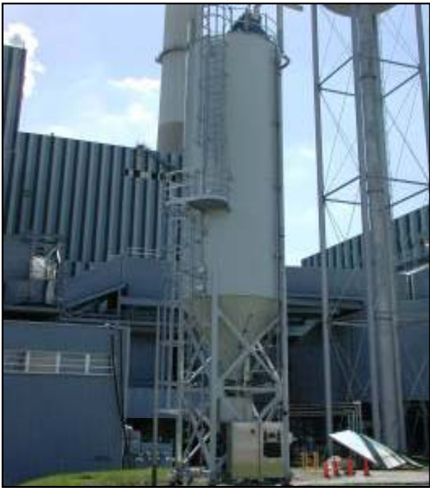
PAC Storage Silo
