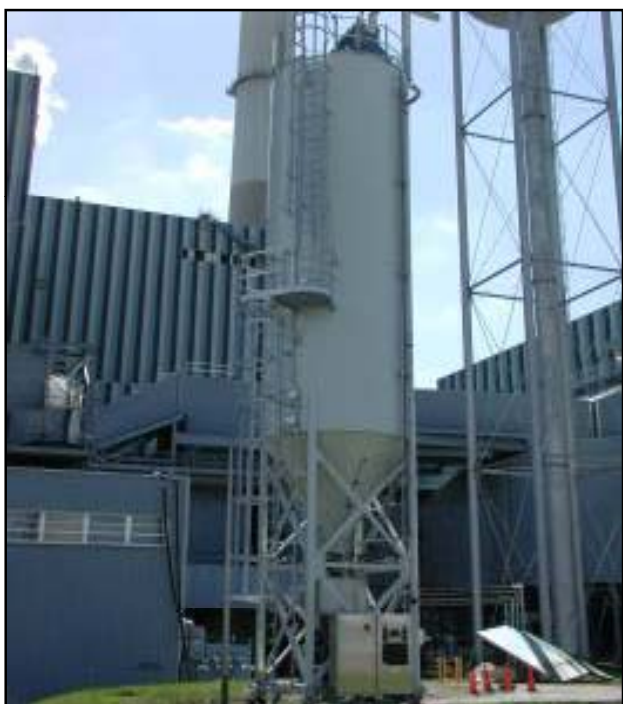
PAC Storage Silo
